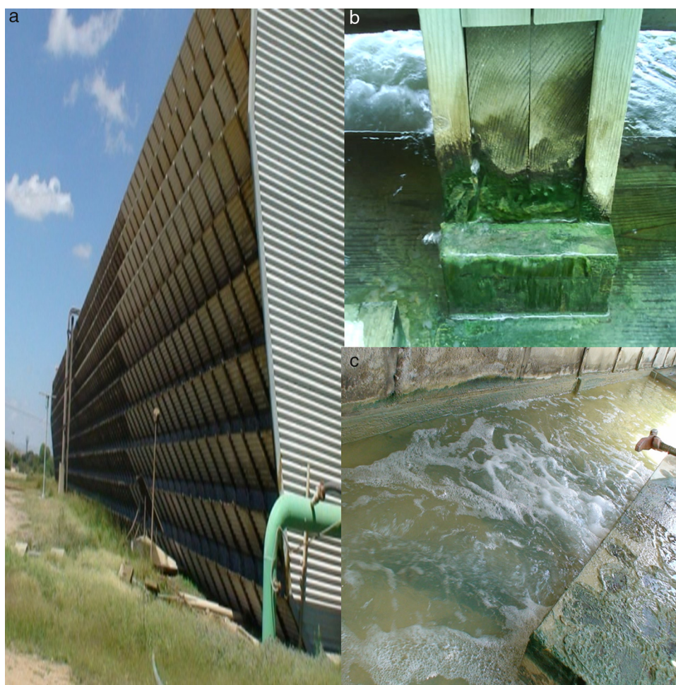
Figure 1. The cooling tower in the thermoelectric power plant of Villa de Reyes, San Luis Potosí, Central Mexico (a). The samples of biofilms composed by microalgae were taken at the top of the tower (b). Floor of the cancels in the top of the tower with microalgal mats, showing the turbulence of the water (c).
